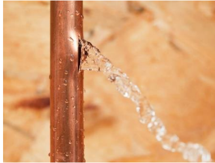
Figure 2. Water Leak in Plumbing ( https://www.ul.com/news/understanding-new-leak-detection-technology ).
