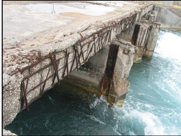
Figure 2. Environmental degradation on a coastal structure.
